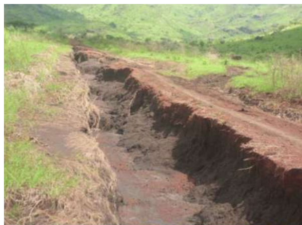
Atar-Mogotio road sections which are badly affected Ngenge sub county
