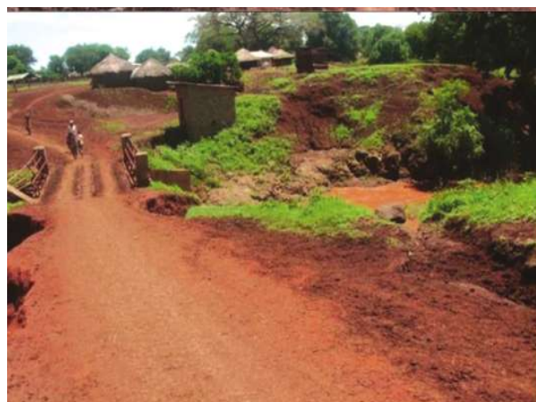
Bridge at Ngenge on the verge of collapse
